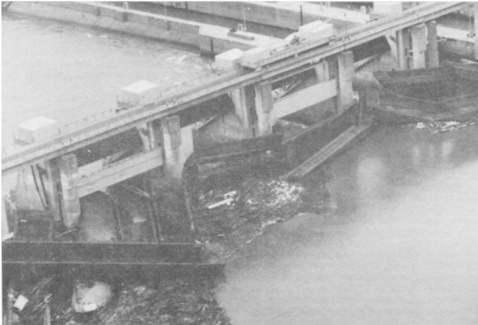
Figure 7-8. Accident at Maxwell Lock and Dam, Ohio River
