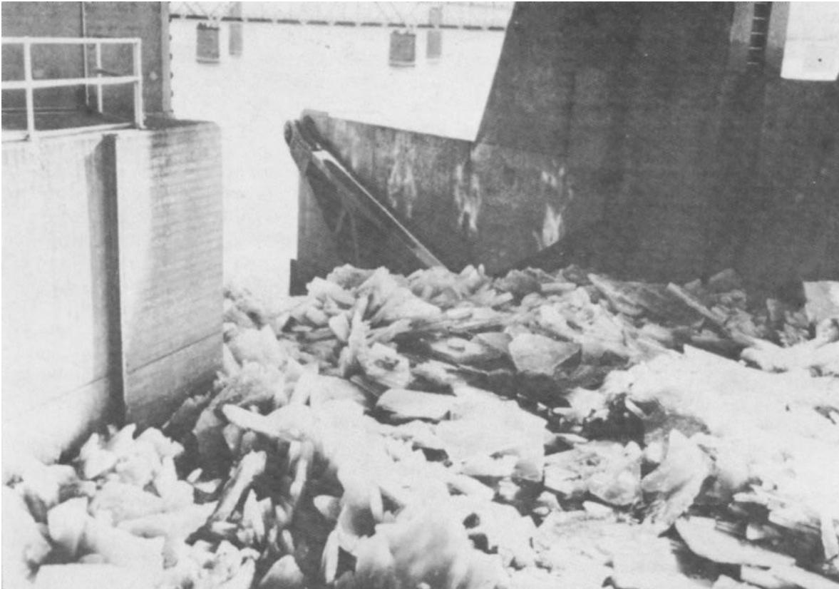
Figure 5-23. Ice on control gate
